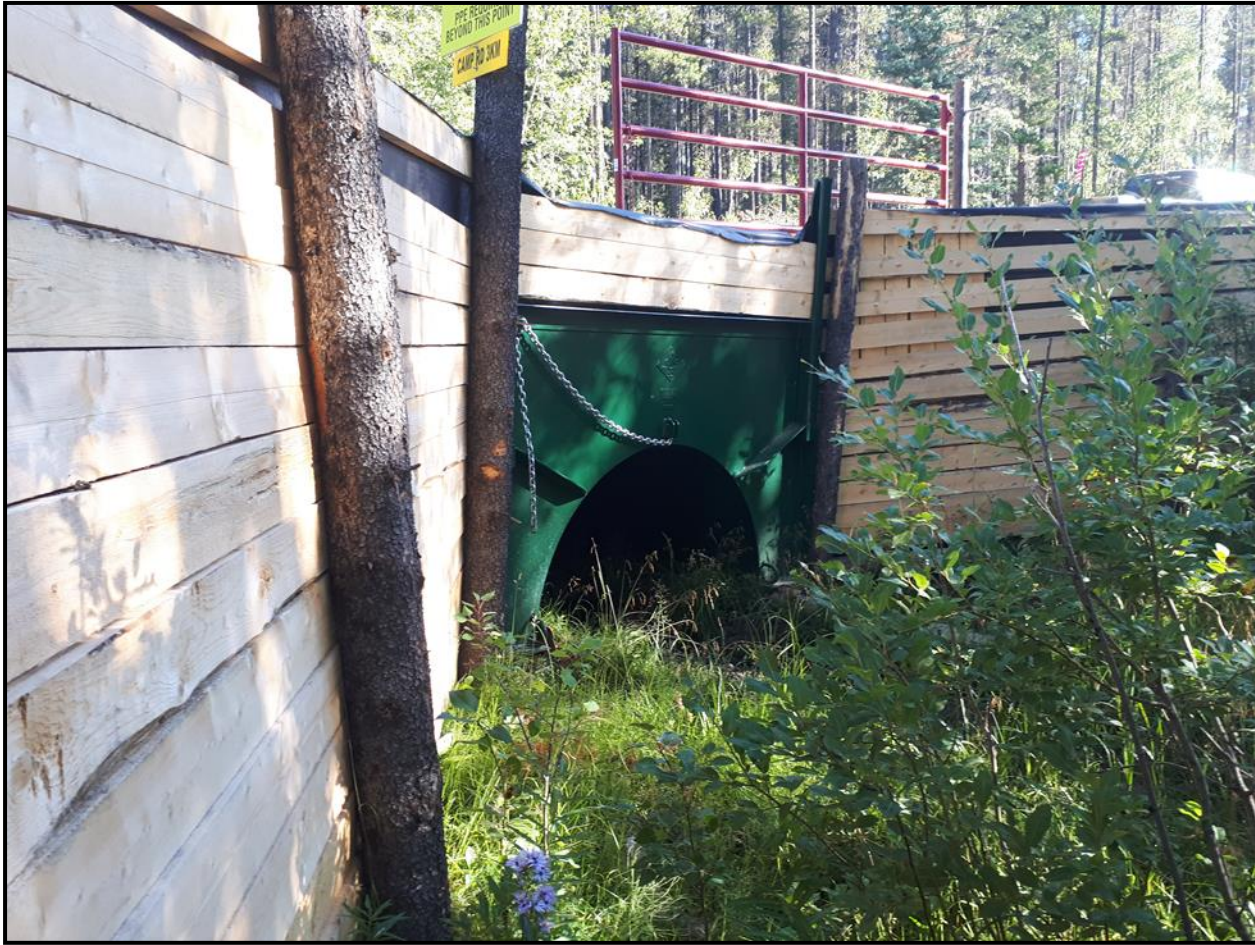
Figure 2. The Company is using more metal arch culverts which a easily installed and reusable.
