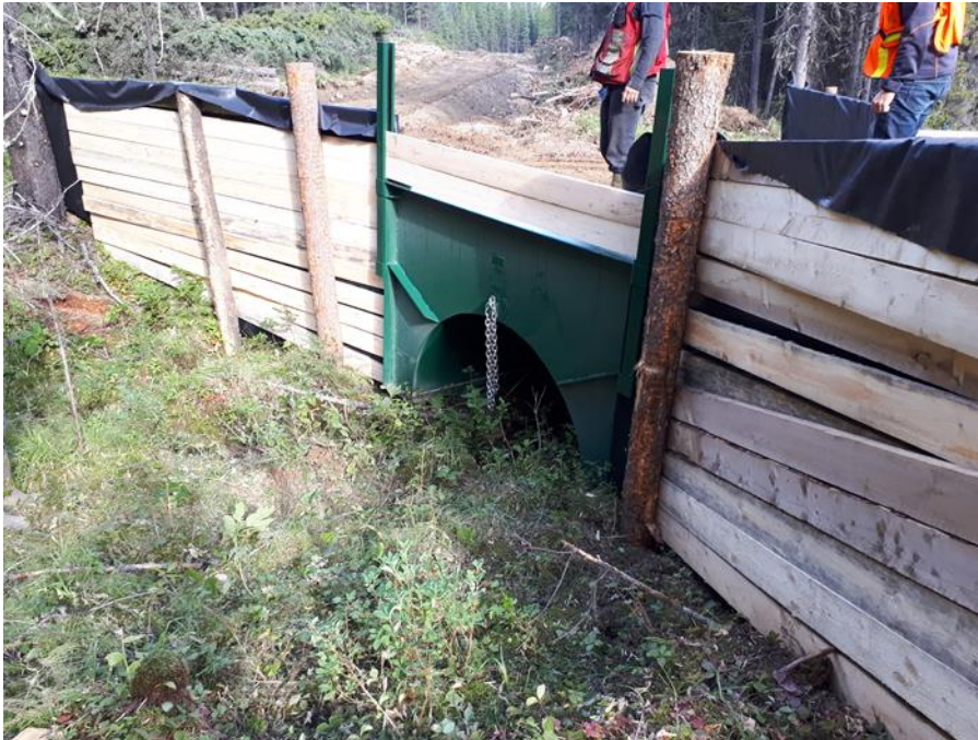
Figure 1. A steel arch culvert installed near Block 1979
